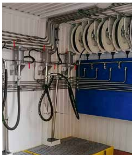
Container de lubrification
