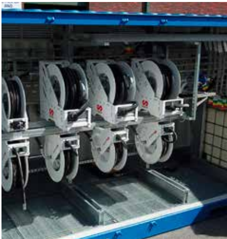
Stations de lubrification
