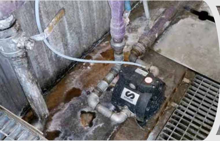
Pompe de process.
